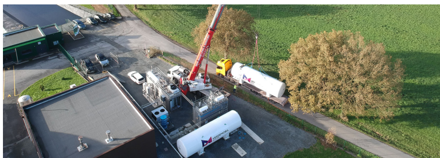
GAZTEAM BIOCO 2 | @VERDEMOBIL BIOGAZ
